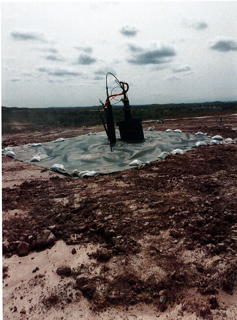
Photo 3: Gas well boot in cap area
