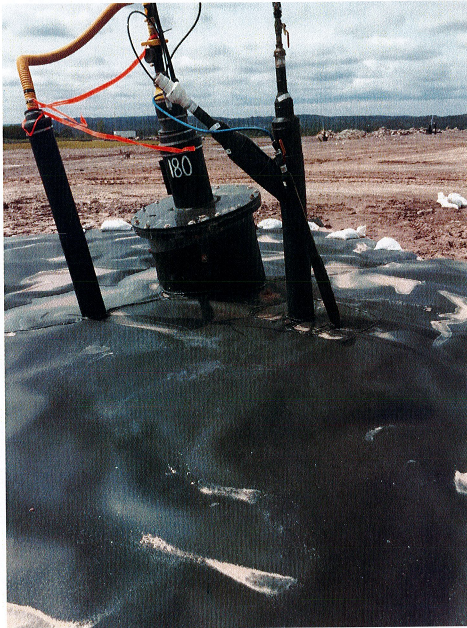
Photo 4: Gas well boot in cap area
