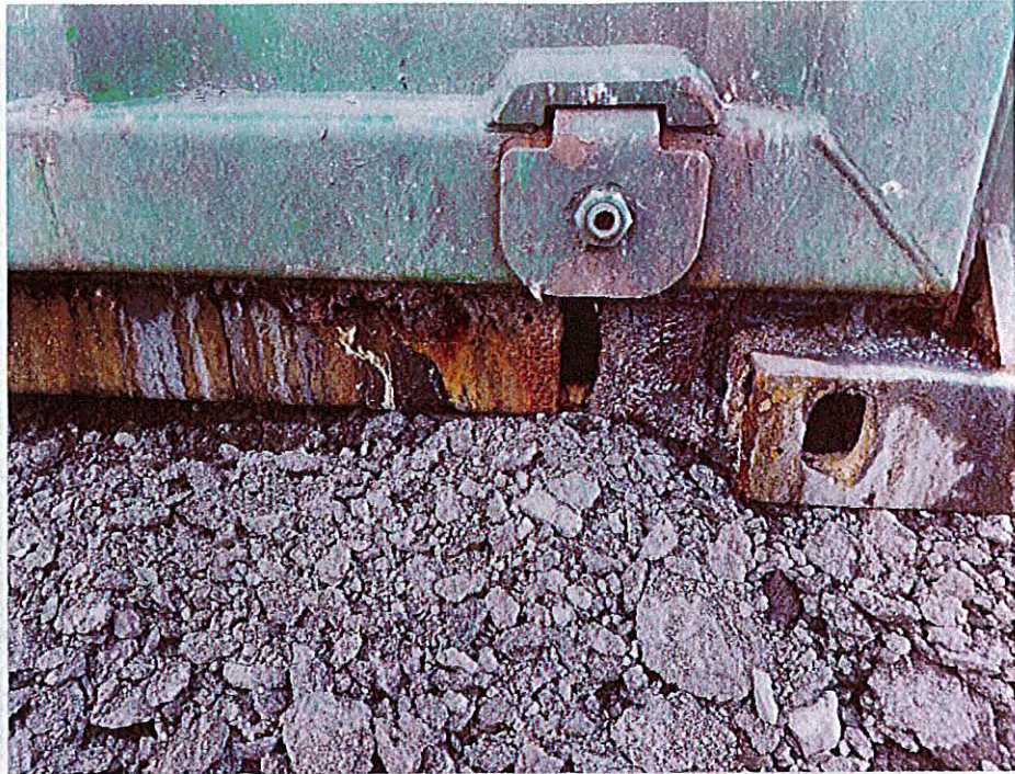
Photo 39 – Varick Rail Container WMNY #9779 –Leaking from bottom right corner of door
