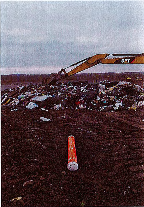
Photo 43 – Retrieval of Temperature Probe from a Varick Rail Container
