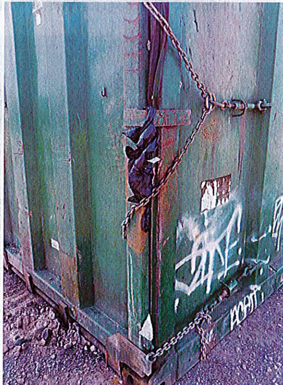
Photo 68 – Review Rail Container USWX #9305 – Right Side of Door
