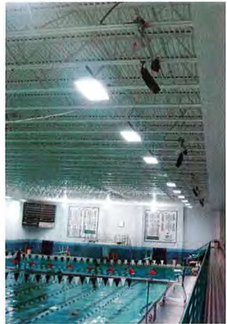
Airius Fans Mounted on ceiling, Rec. Center- Fort Collins, CO
