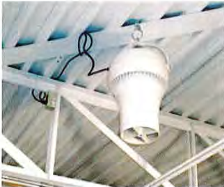
White Airius Fans on Ceiling
